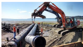
Installation of a pair of 42-inch storm drain outfalls into Oak Harbor Bay.
